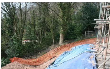
Orange webbing used as protective fencing is not acceptable
